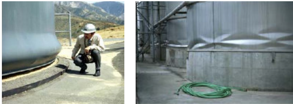
Figure 2: Elephant Foot (L) and Diamond Shape Buckling on a Tank (R) (Malhotra, 2006)
