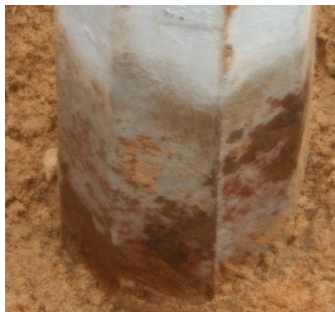
Figure 1 Example of S5 pole condition after excavation and cleaning
