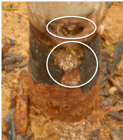
Figure 2 Example of S1 pole condition after excavation
