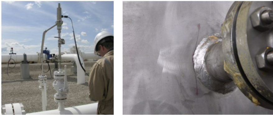
Figure 1 Example photos of SBC attached to mainline piping (left) and FIV fatigue crack at SBC weld to mainline (right) (Wood Beta Machinery, 2022).
