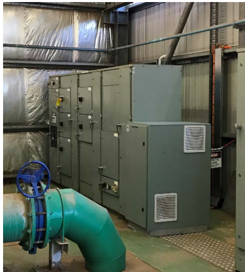
Figure 1 Electrical switchboard in water pump station
