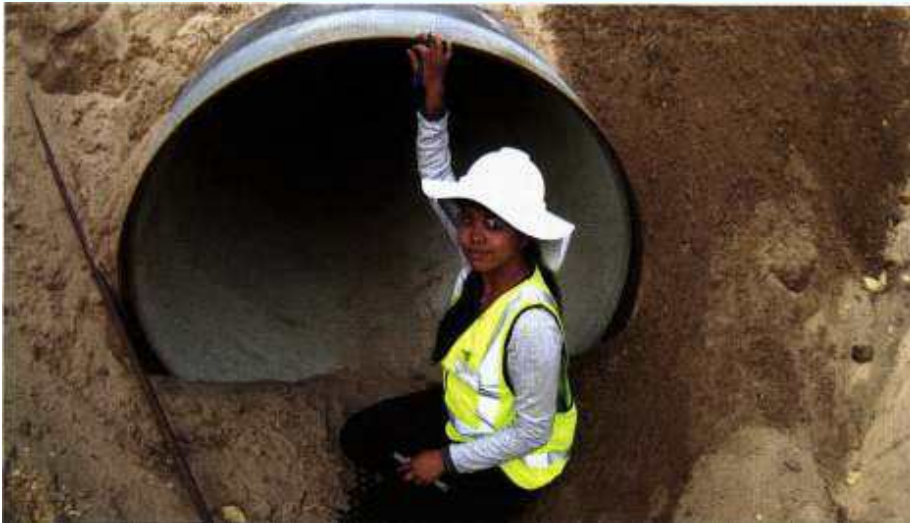
CEED student Shruti Gupta investigating the effect of site operations on buried pipe integrity.
